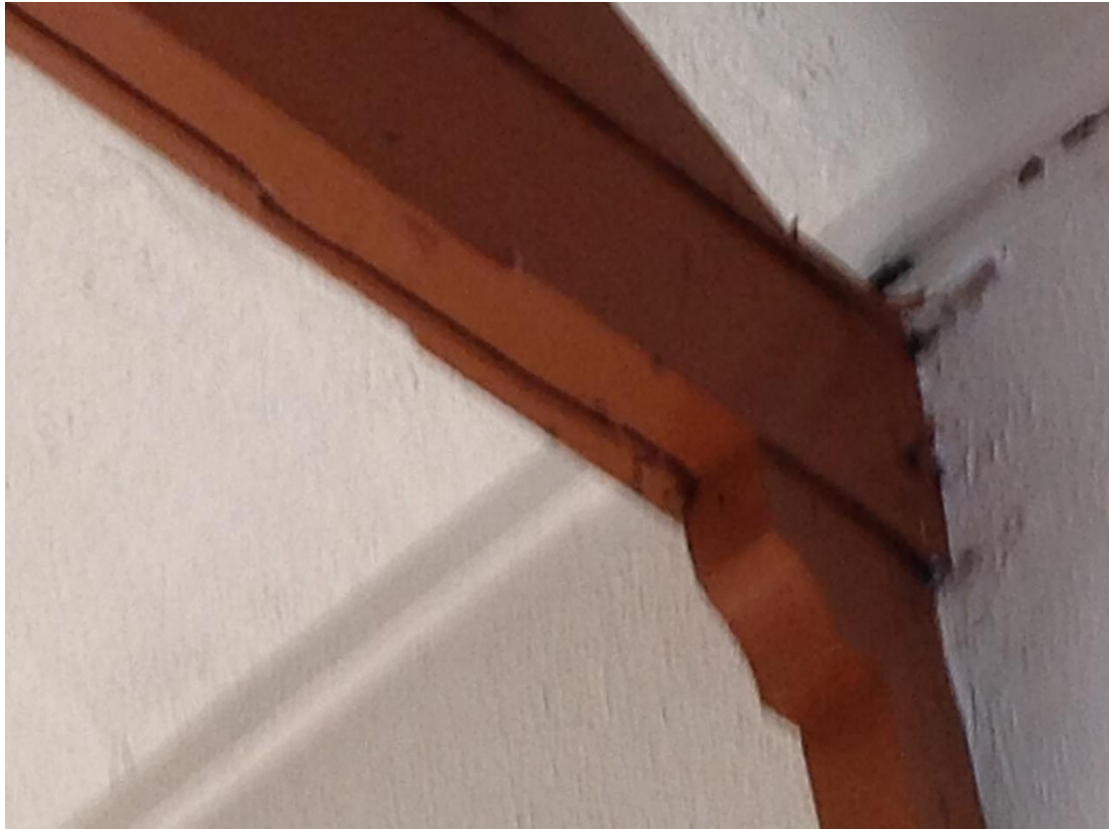
Image 6: Shows cracking in roof joists.
