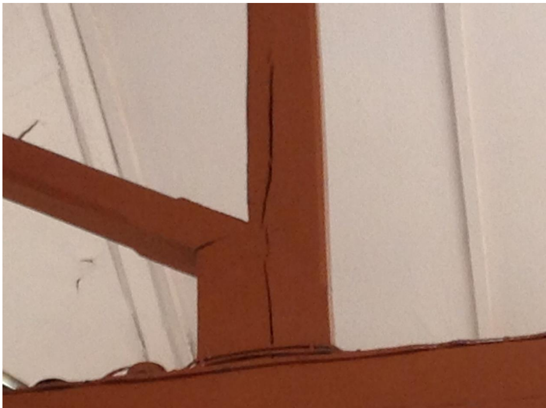
Image 7: Shows roof joist supports cracking.
