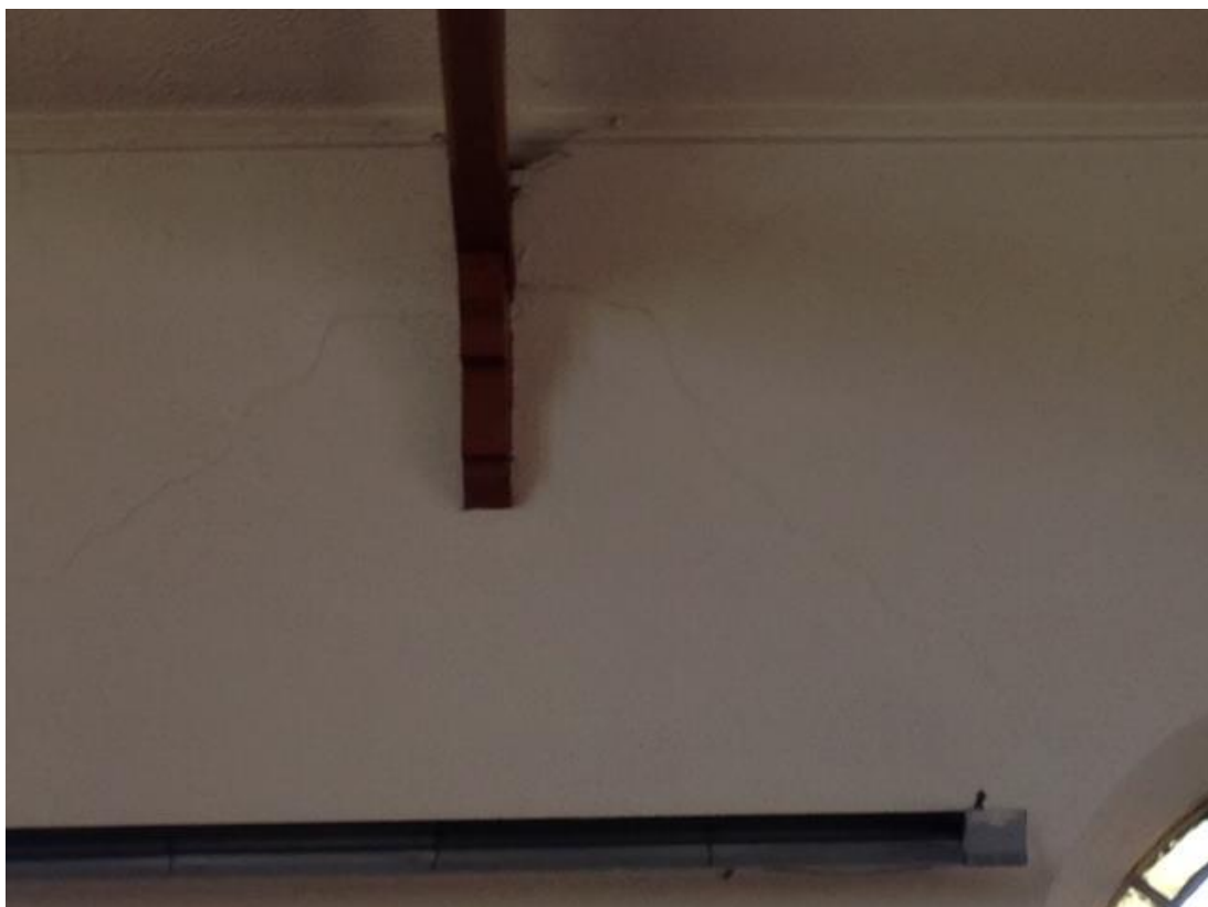
Image 5: Shows wall cracking under weight of roof having effect onto windows.
