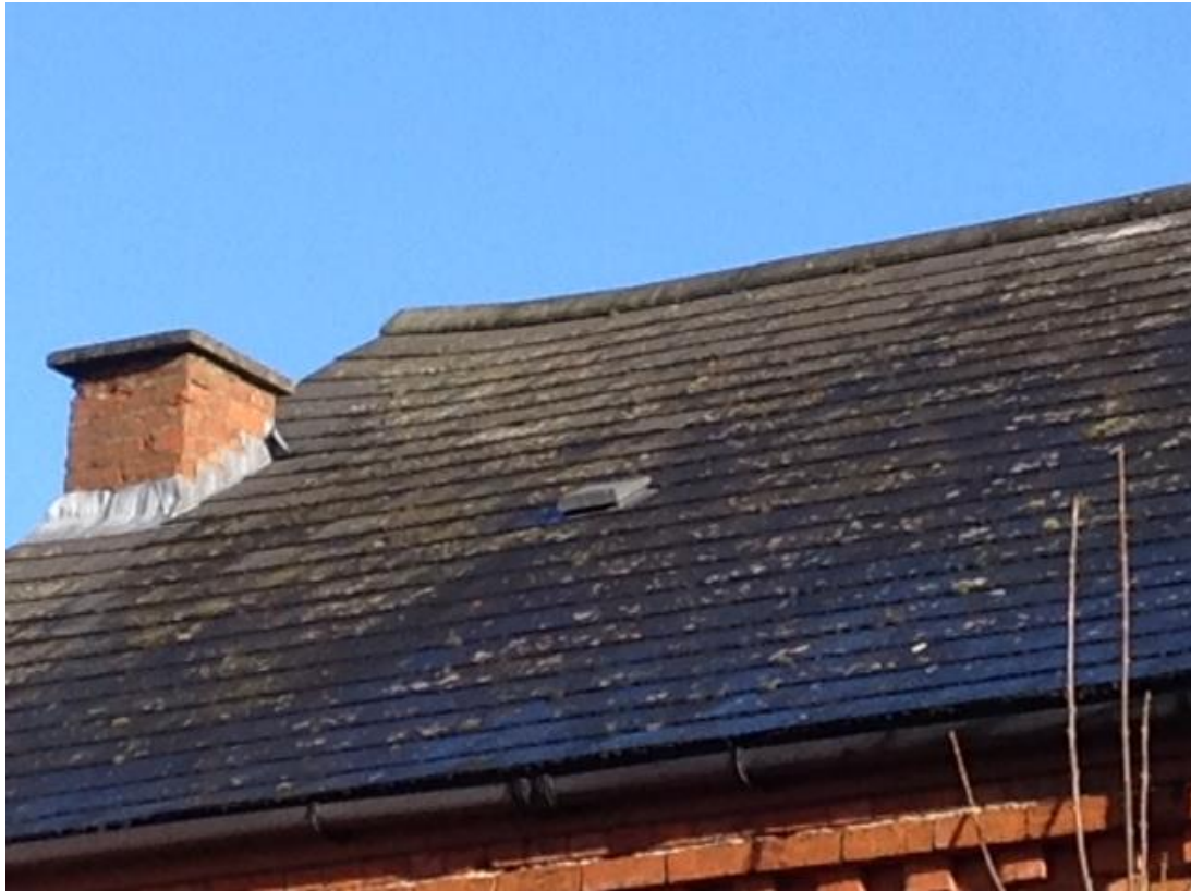
Image 8: Roof line shows a dip.
