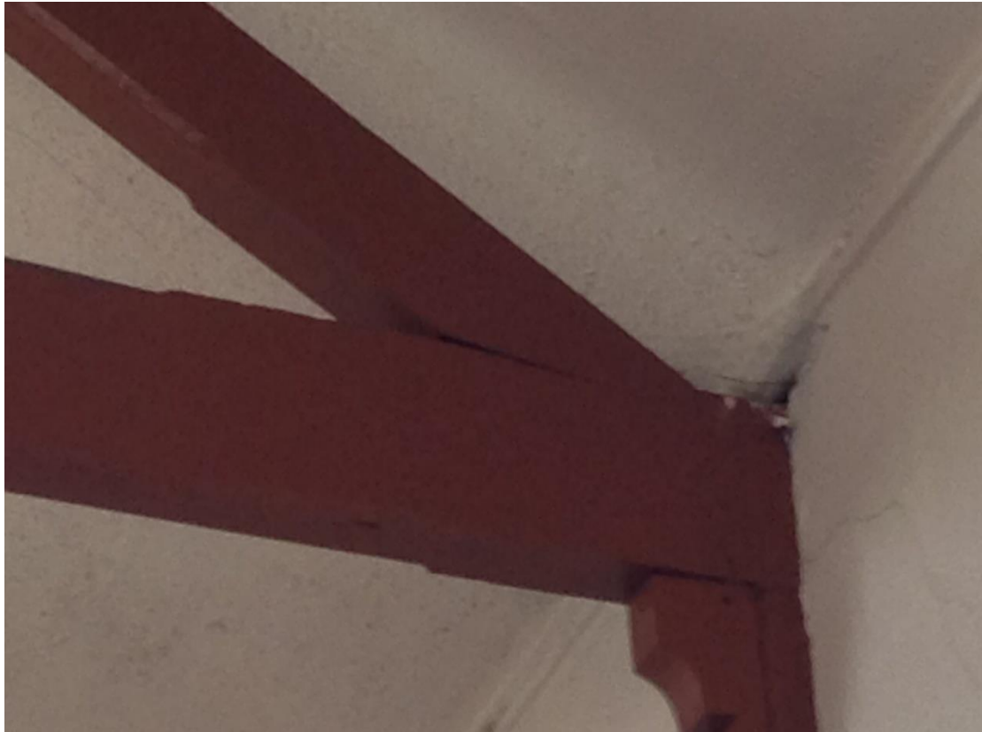
Image 4: Joist showing signs of movement and spread.
