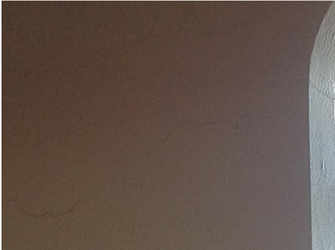
Image 2: Shows gable end wall cracking.
