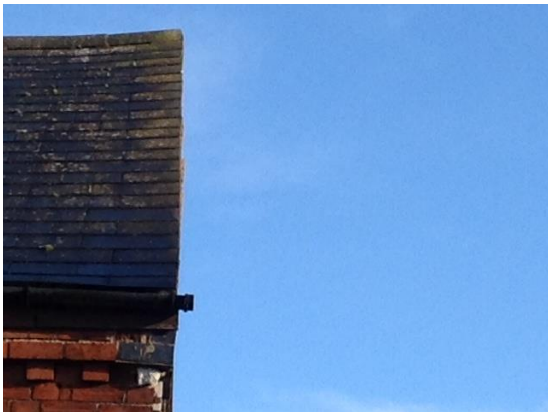
Image 9: End gable showing signs of movement.
